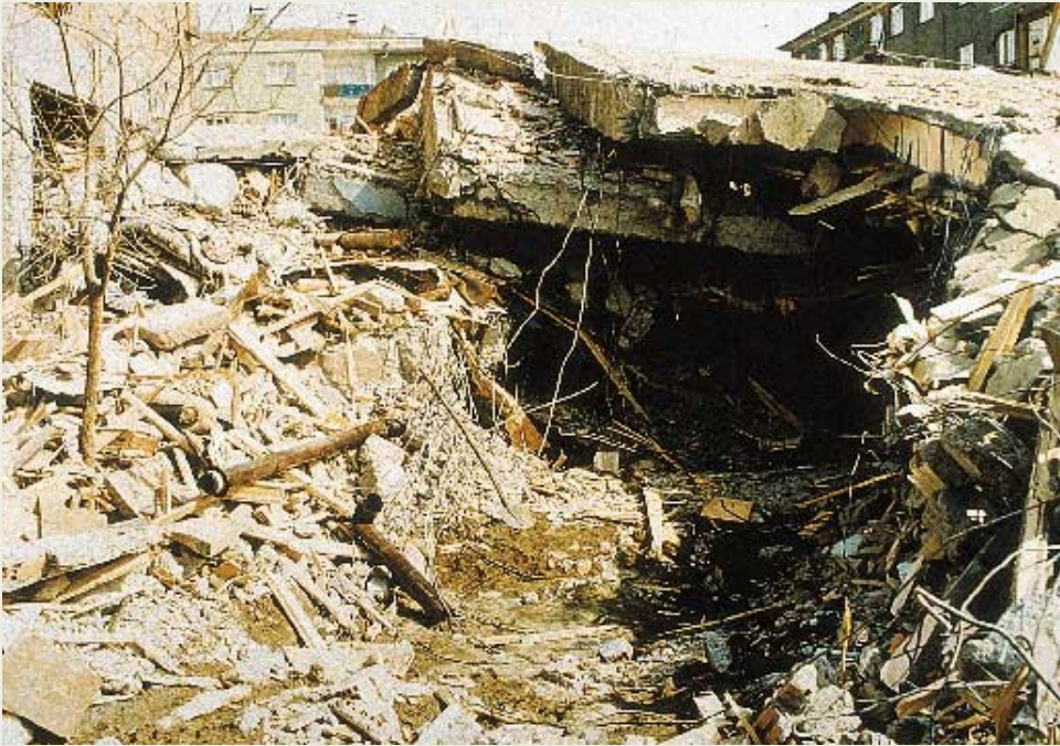
Photo 15: Creating a wide penetration front by removing all materials from the facade of the building. (Frontal Penetration)
