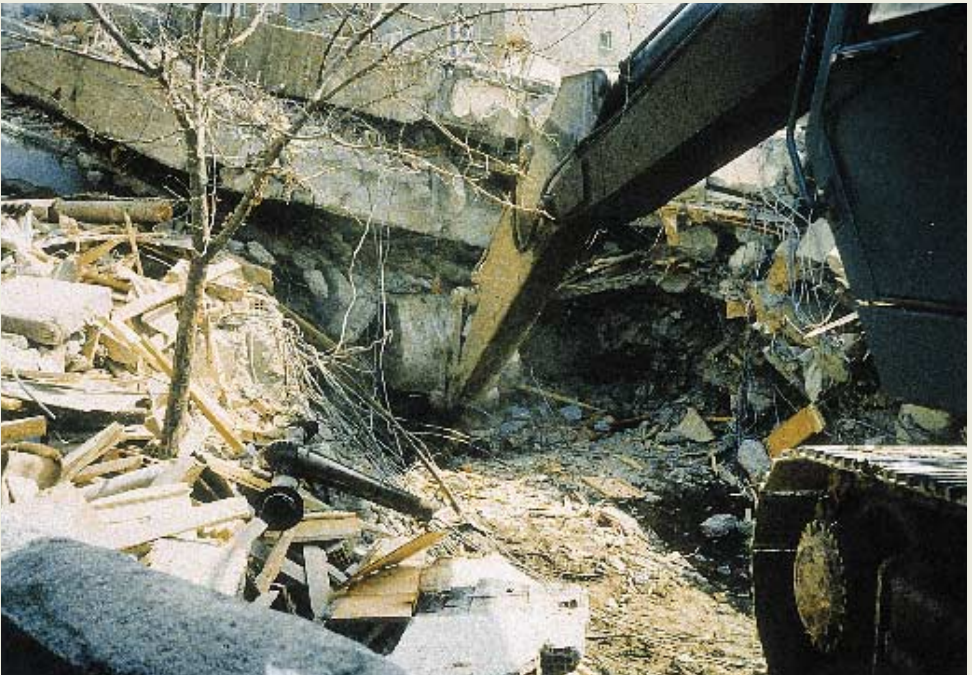
Photo 14: Creating a wide penetration front by removing all materials from the facade of the building. (Frontal Penetration)
