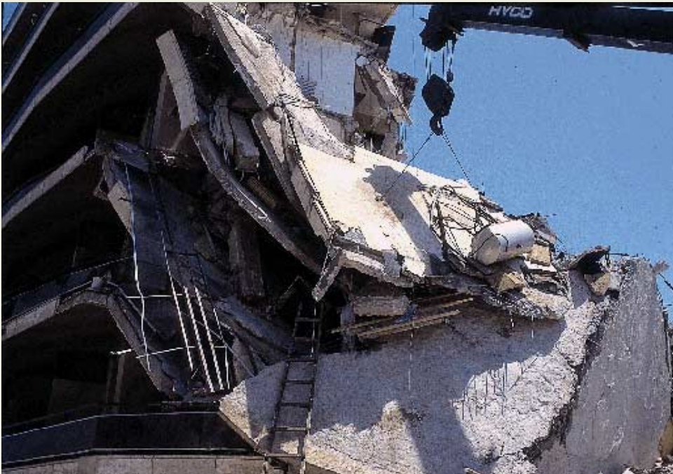
Photo 11: Lifting by using a crane, a big part of a slab that had a steep inclination because of the building's partial collapse. Cutting off this part from the rest of the slab by cutting the reinforcement across the fracture lines of the slab. (Aegio 1995)
