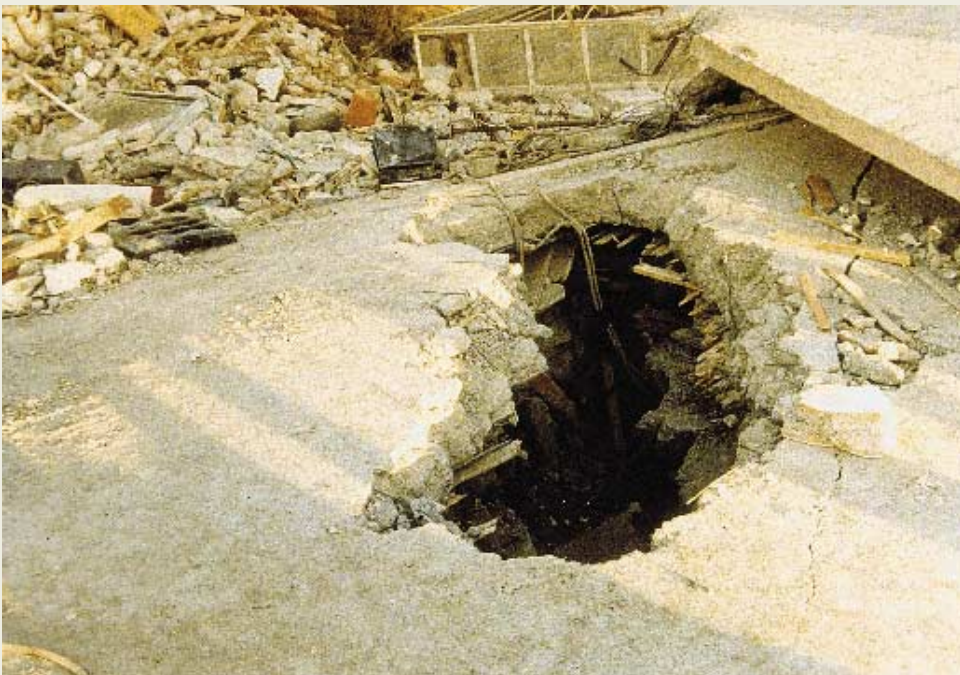
Photo 12: Starting point of a descending penetration on a location where the slab has rather low inclination, in contrast to the left side where the inclination of the slab is steeper. Two slabs were penetrated and horizontal penetration followed, downwards to the point that the arrow indicates. An infant was rescued 24 hours after the earthquake. (Rescue Operation, Kalamata 1986)
