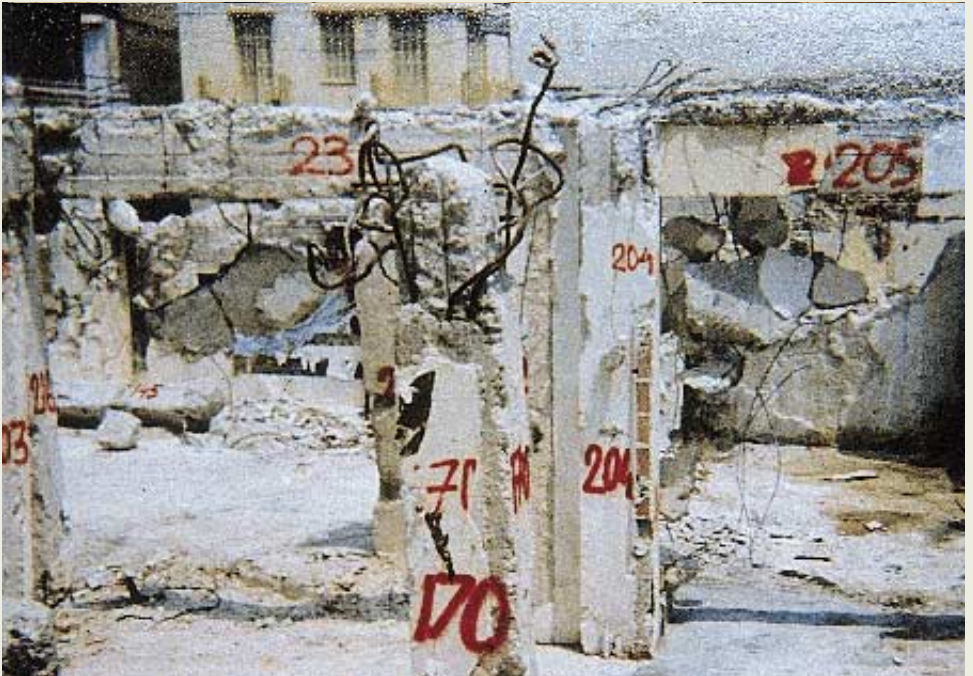
Photo 1: Beams and columns of the basement. Geometry is maintained even though six floors have totally collapsed above them. Apart from a survival space there is also enough space for a vertical ascending penetration to be undertaken. (Investigation work, Loutraki 1981)
