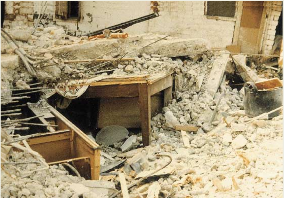
Photo 2: The table, apart from some slight damages on the upper part, has maintained its geometry and underneath there is space void of construction materials. Ideal shelter during an earthquake. (Kalamata 1986)
