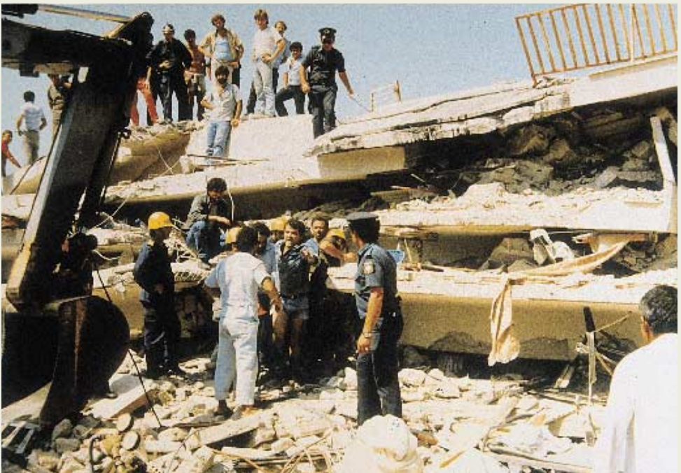
Photo 5-6: The first stage of the operation is in progress; cutting a part of a R.C. beam and slab of the floor under investigation. Contact with a trapped person located 3 ~ 4m away from the facade. During the second stage, horizontal penetration was applied. Furniture and walling material had to be splitted and removed in order to reach the trapped person. Duration of the operation 3 ~ 3.5 hours. (Rescue Operation, Kalamata 1986)
