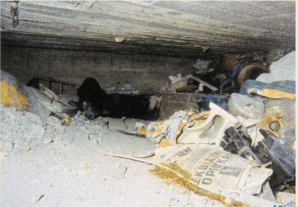
Photo 13: Pilots of a building that has totally collapsed. Even though there is a lack of walls, there is enough space not only for survival but also to start an 'ascending penetration'. (Training in Ruins, Kalamata 1986)
