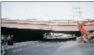
Collapse of a flyover part of a highway (Northridge earthquake, California 1994)
