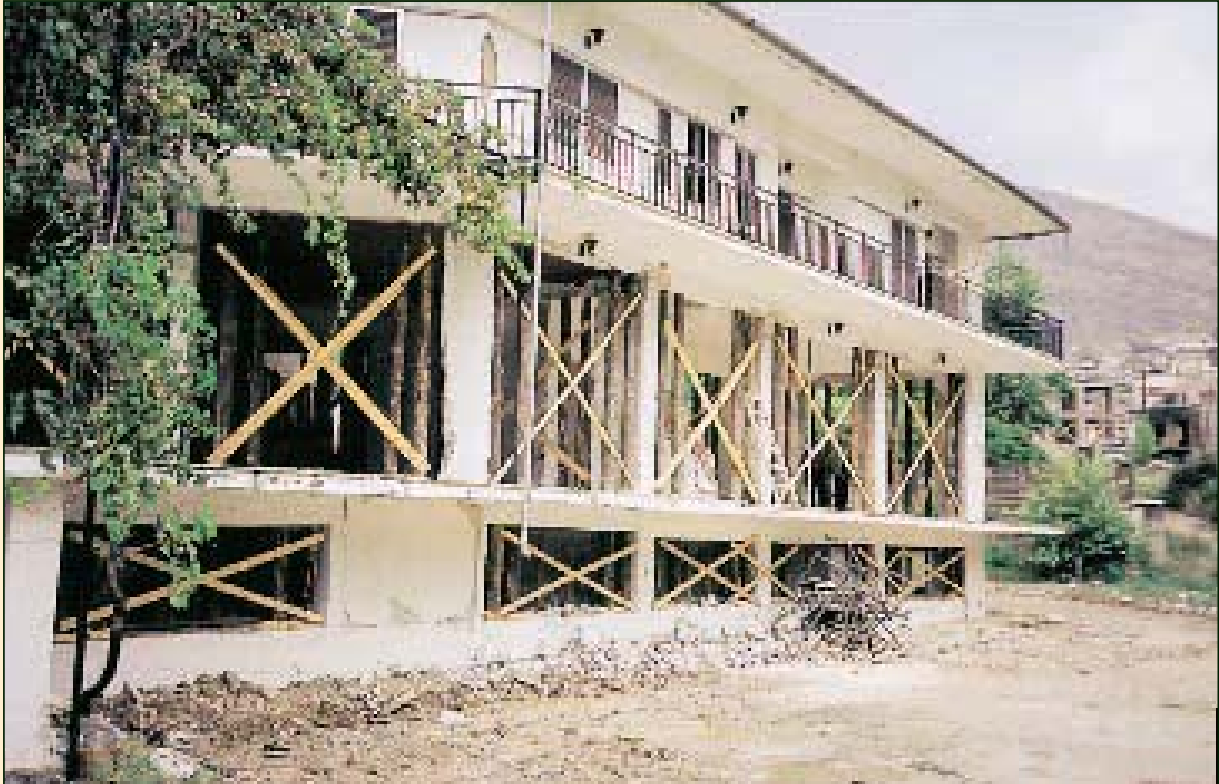
Extended propping using tree trunks. The propping has been applied on the ground floor and basement.
