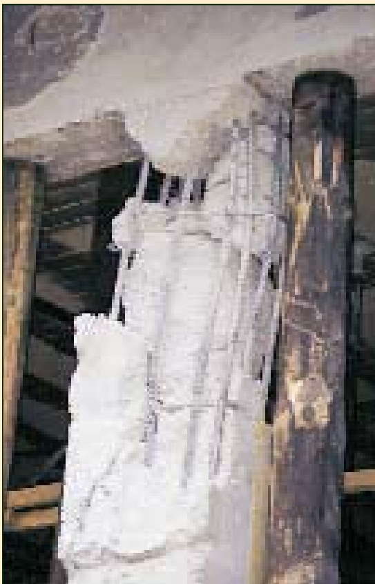
Detail of propping with tree trunks on heavily damaged column.
