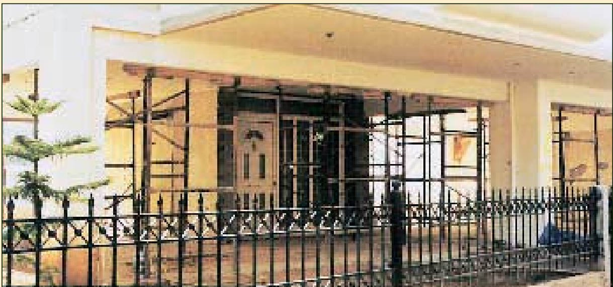
Attika – New Herakleio 1999 Extended propping using whole sections in pilotis with heavy damages on many columns.
