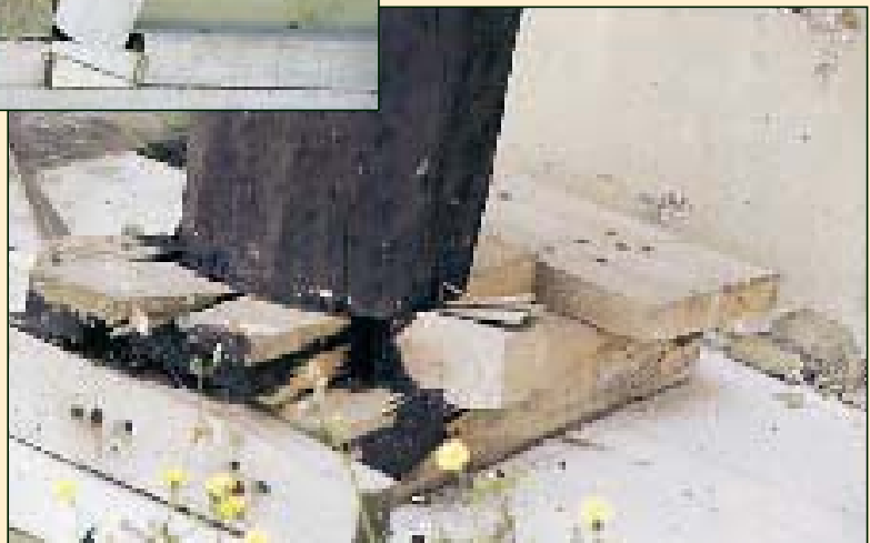
Wrong wedging on tree trunk propping.
